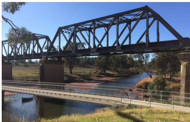
Old Railway Bridge and Shibble Walking Bridge, connecting both sides of the Macquarie River at Dubbo.
